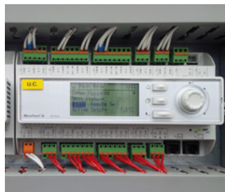
Controller box upgrade
